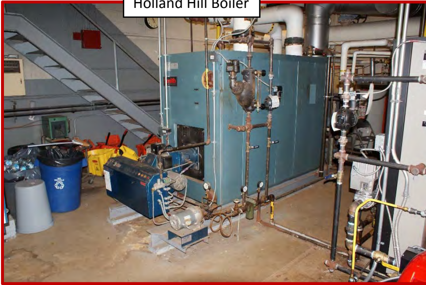
Holland Hill Boiler
